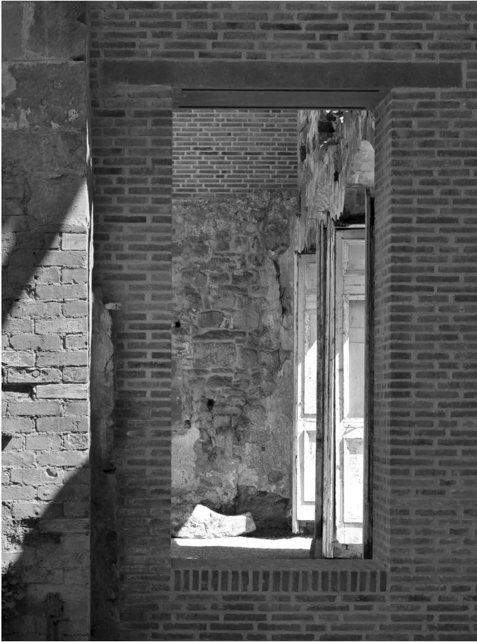
New brickwork and concrete lintel, binding and buttressing the remaining stone walls
